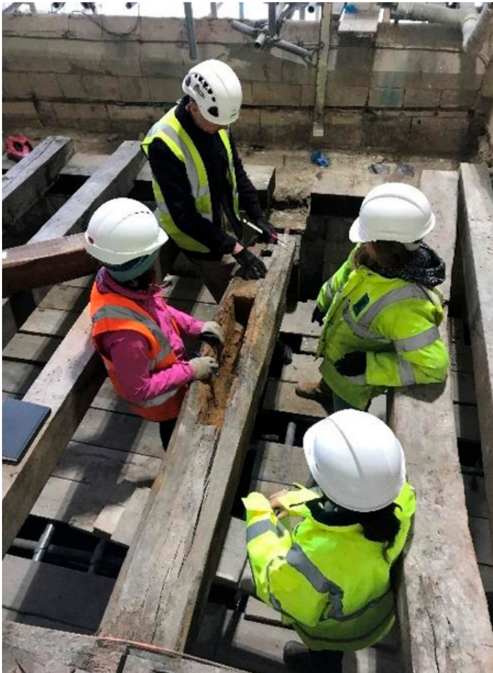
The medieval truss damaged by rot and insect infestation
